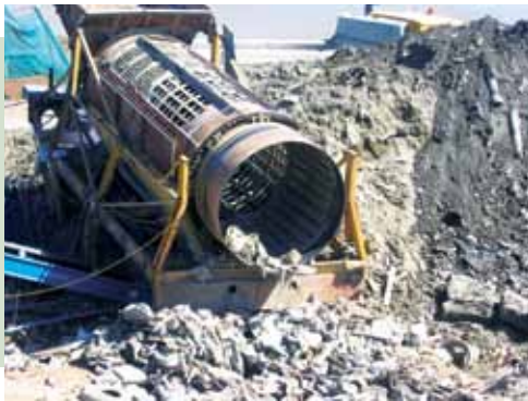
A rotating screen separates refuse and debris from the soil and gravel in materials excavated from the site
