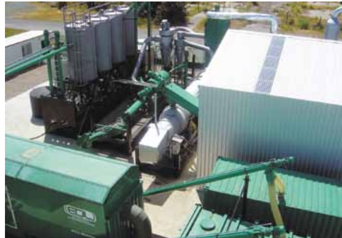
The EDL plant
